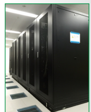
Fig. 2. Seismic Server Racks
